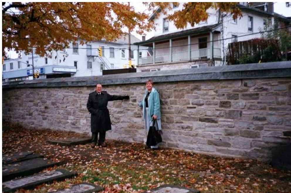
Doug and Marianne Thompson in front of restored wall. Photo courtesy of Marianne Thompson
